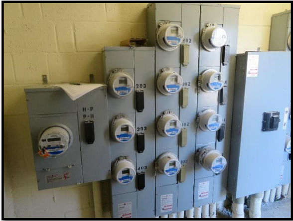
Main electrical panel and meter banks
