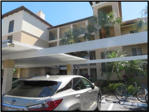
Carport with missing roof
