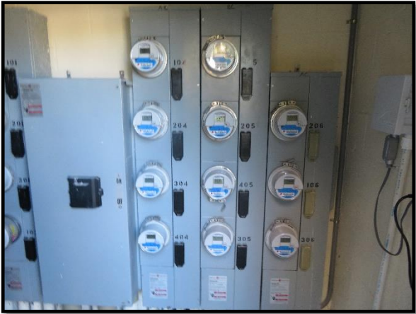
Main electrical panel and meter banks
