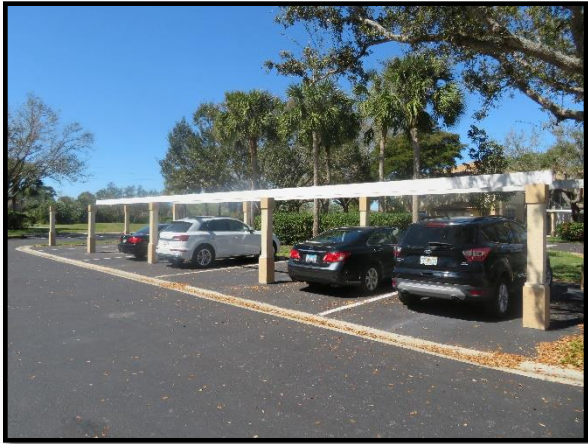
Carport with missing roof
