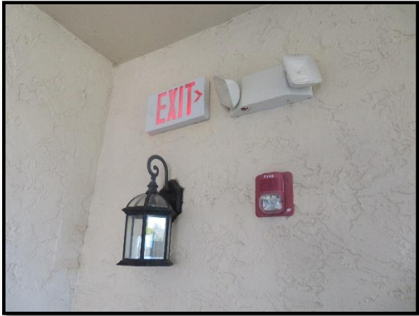
Exit sign, emergency lights and annunciation device
