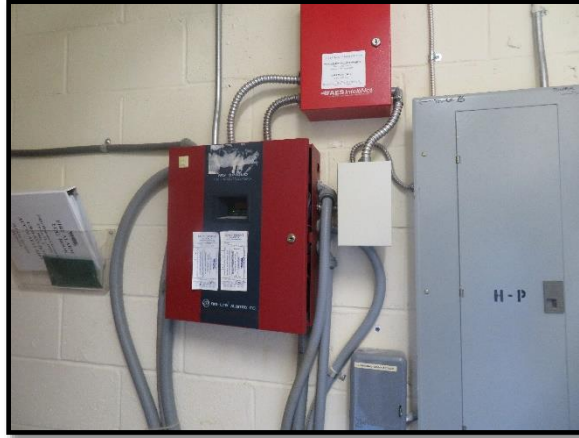
Life safety system control panel
