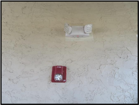
Annunciation device and emergency lights
