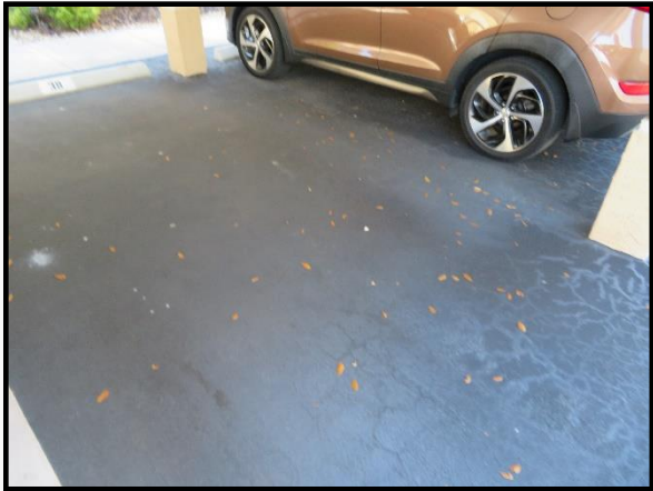
Asphalt pavement with surface cracks evident
