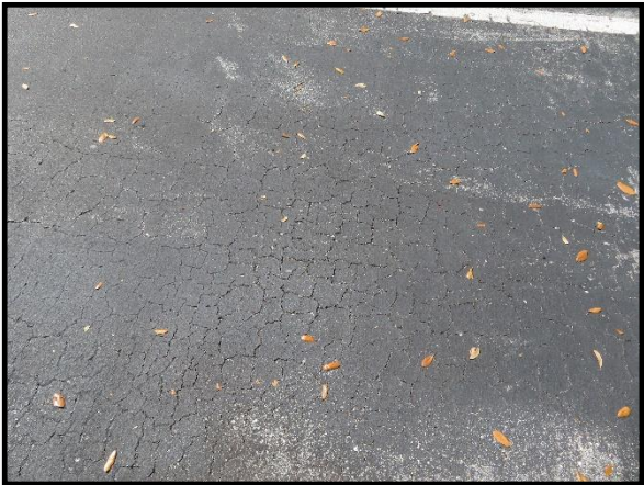
Asphalt pavement with surface cracks evident
