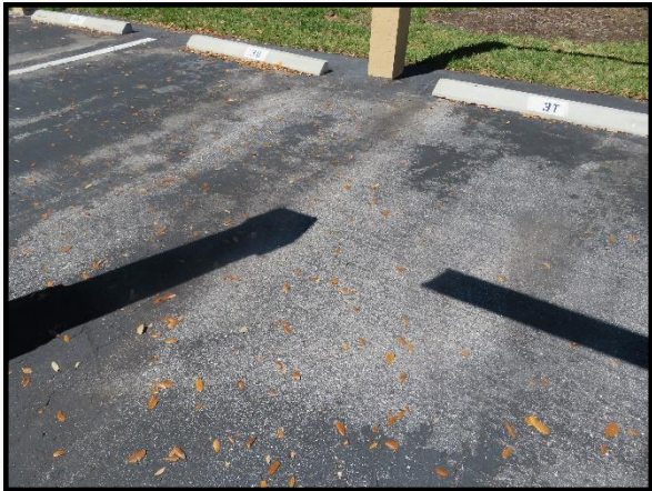
Asphalt pavement with surface deterioration evident
